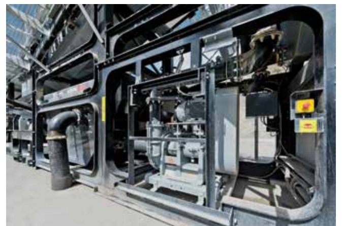
Centrifugal Pumps, Roll out for Service Access
