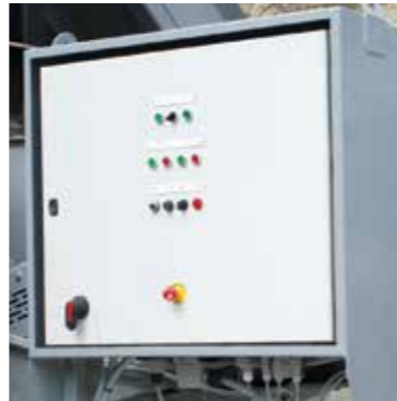
H12 Feeder Control Panel
