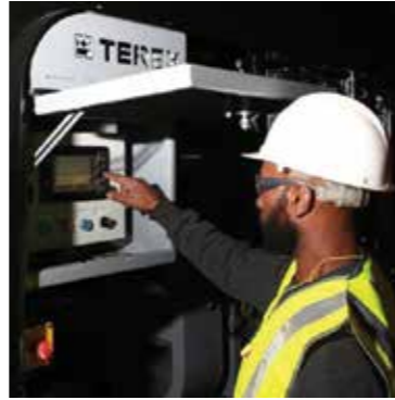
Aggresand™ Control Panel
