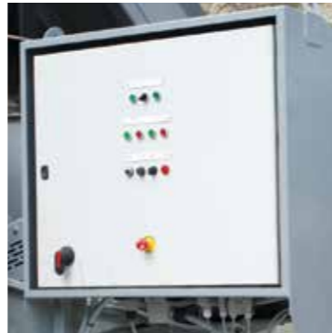
H12 Feeder Control Panel
